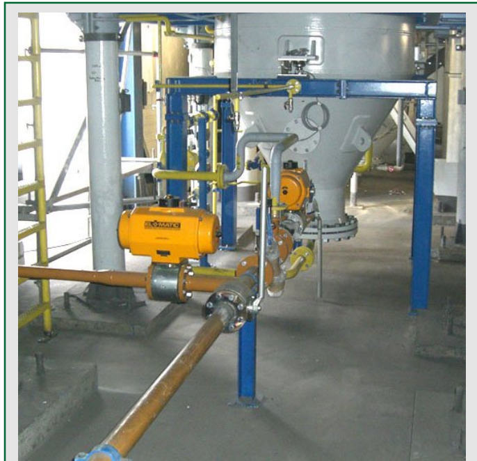
Intermediate conveying equipment
