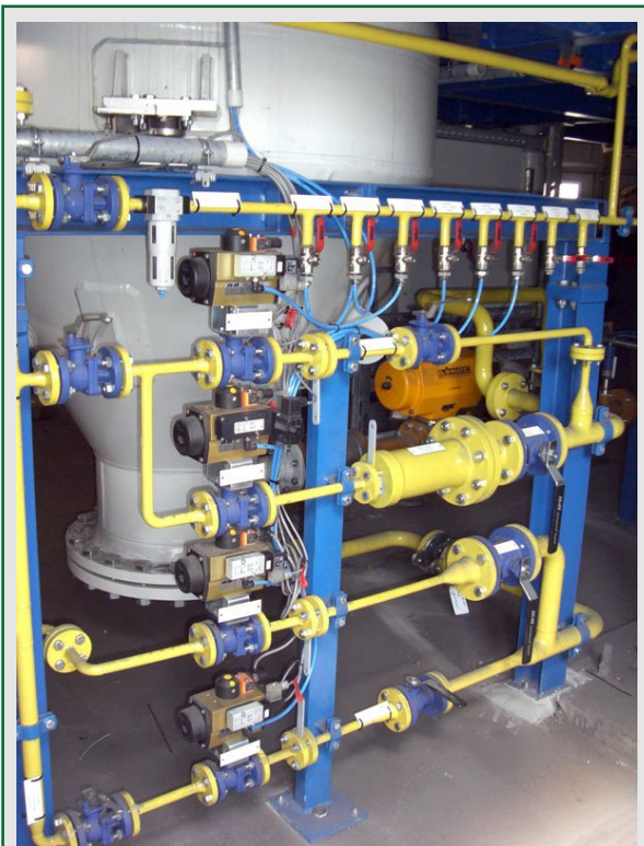
Valve terminal intermediate conveying plant
